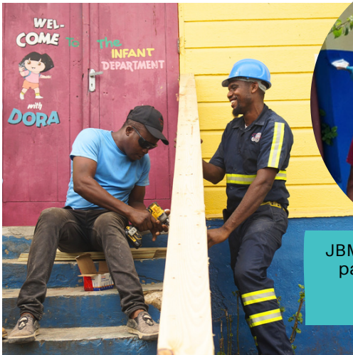
Port and Lydford Maintenance team members, Terrence Moody and Jermaine Cole, installing a staircase at Sturge Town Primary
