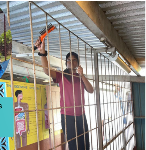
Project Officer, Malika Pottinger, prepping the roof and grills for painting at Waltham Abbey Primary
